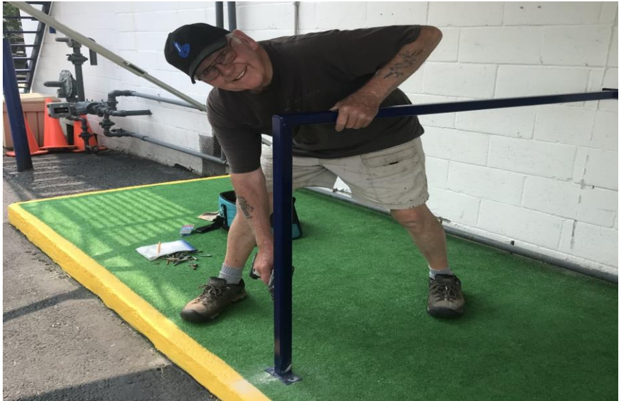
Paul Penney, House Chair installs a safety railing on the patio step outside the patio door.
